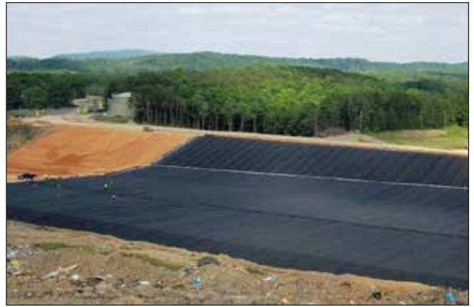
Textured Landfill Liner
